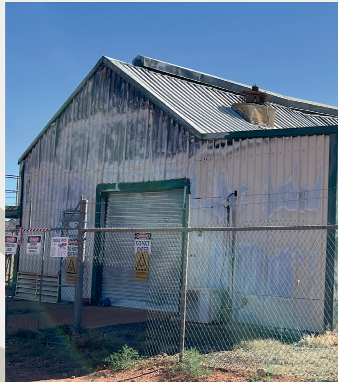
Replacement of this temporary power station to a hybrid solution is underway.
