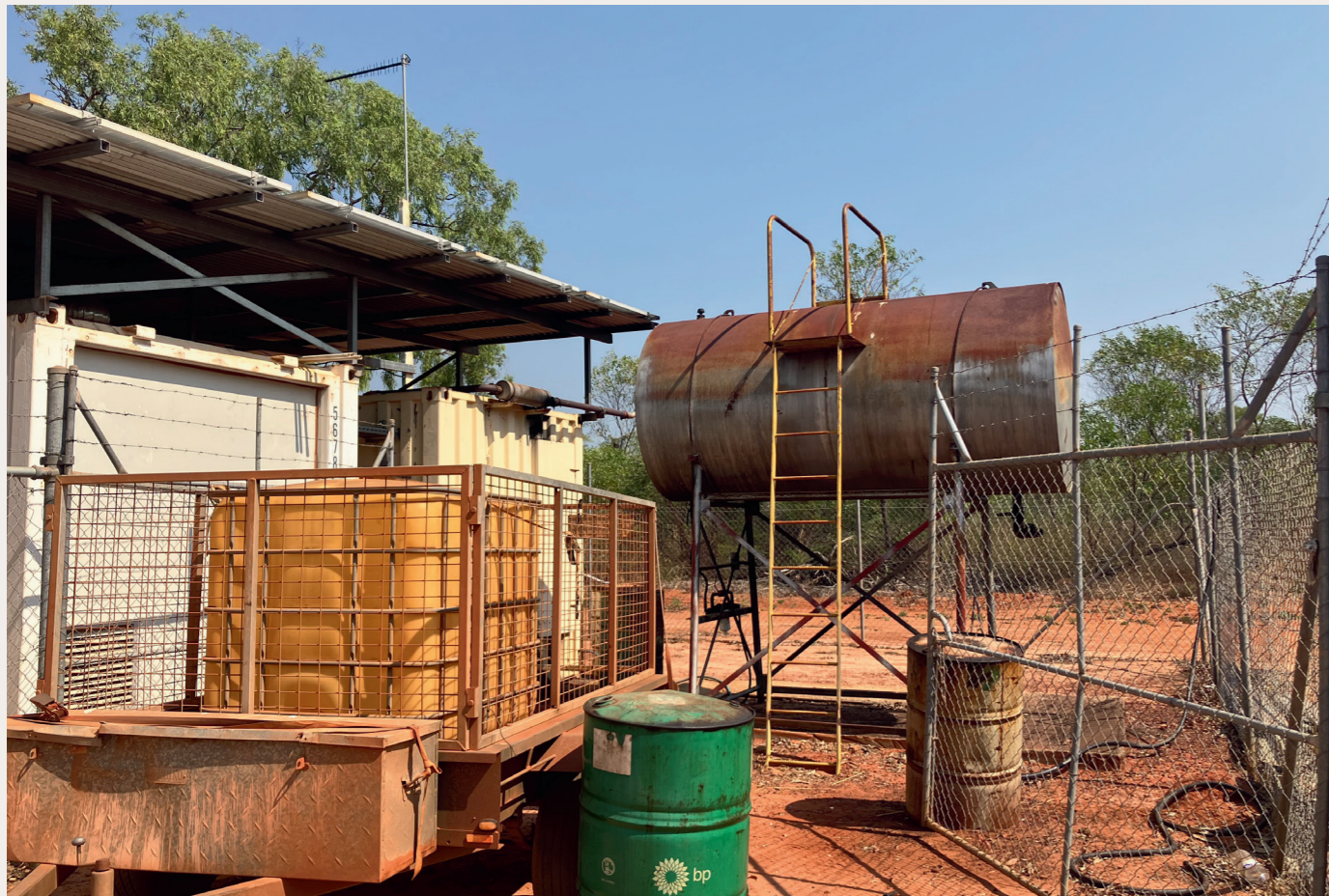
Power assets in a remote community
